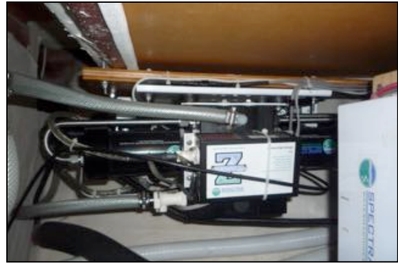
Water maker and treatment system
