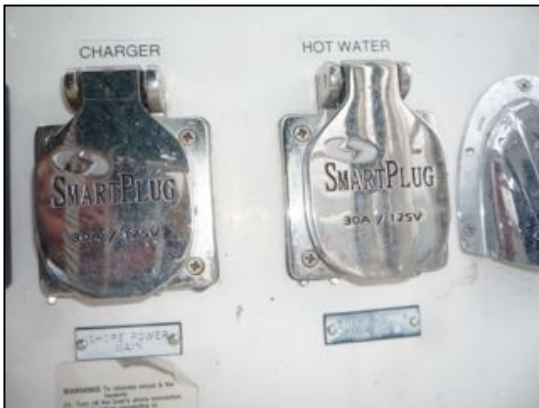
Upgraded shore power inlets
