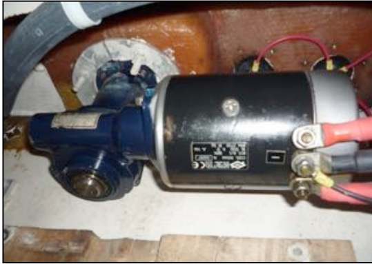
Anchor windlass gearbox and motor
